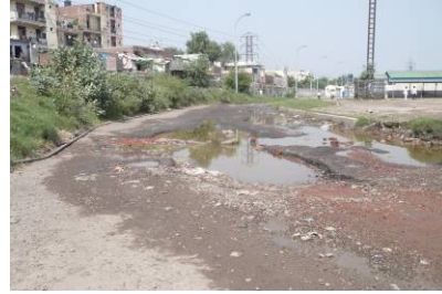
Poor drainage condition
